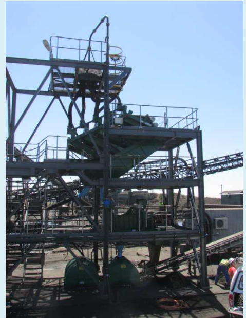
Screening section of the plant
