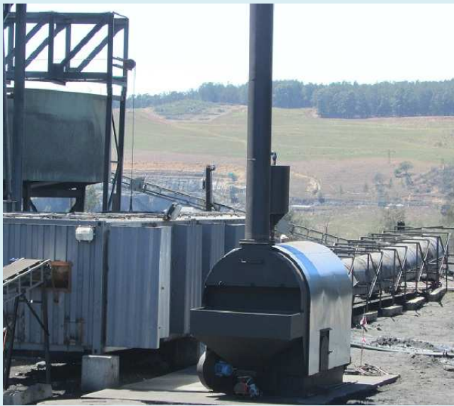
Boiler, Curing Oven and Curing tunnel
