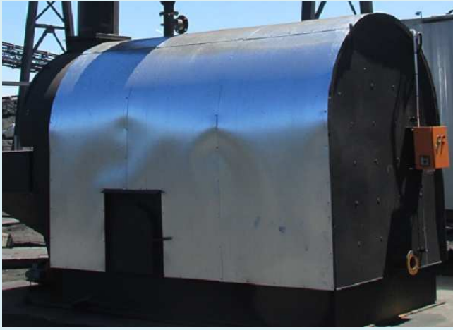
Boiler or Hot water kettle
