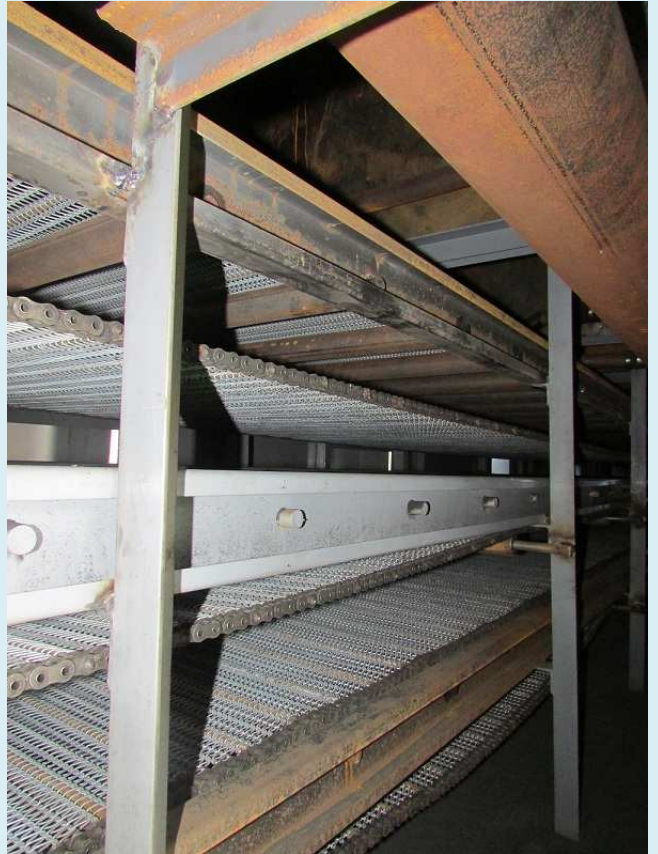
Inside of the curing oven
