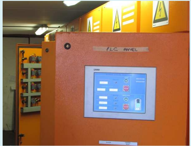
PLC (process control) and MCC (Electrical panel) unit
