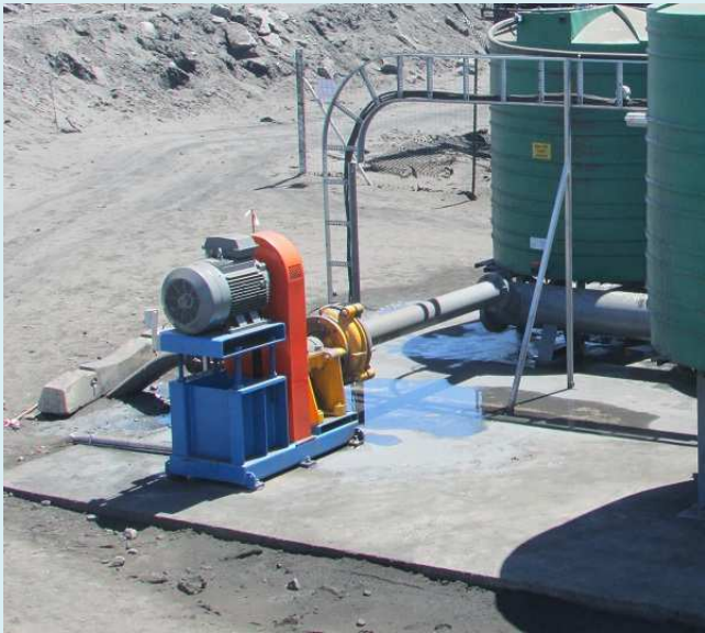
Discharge sump and pumps
